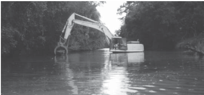
Excavator placing habitat logs with boulders attached by steel cable into deep pools for fish habitat. [Dale Watson]
