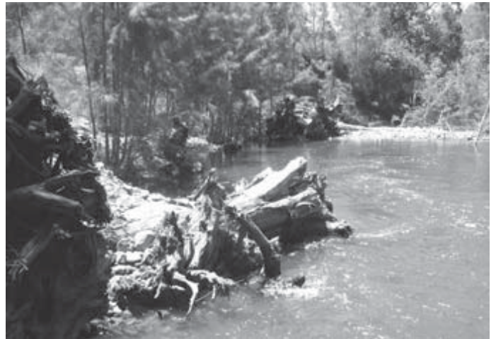
The first of three engineered log jams constructed at Amamoor Creek to protect the bank from further erosion. [Dale Watson]
