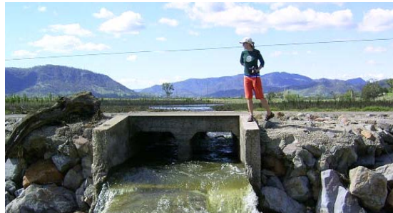
“Worst causeway in the world award goes to: Pages River, Hunter River catchment”. Two small culverts are used to pass water from a river 50 metres wide. Note the ‘waterfall’ on the downstream side, darkened tunnel, white water and increased water velocity. The riparian area is denuded of cover from riparian vegetation also.
