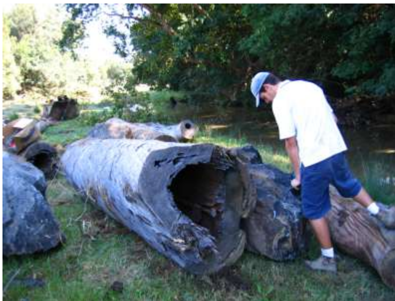
Above: Dale Watson drilling into rock at the Amamoor large woody debris project site
