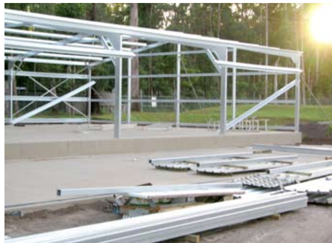
Construction proceeds on the new fish hatchery at Lake Macdonald. [Photo: Vince Collis]
