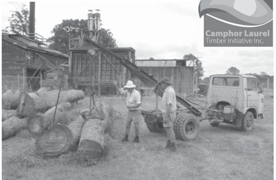
Col Gunson and Stan Ryan relocating a camphor log prior to shed construction. [Photograph by Phil Moran]
