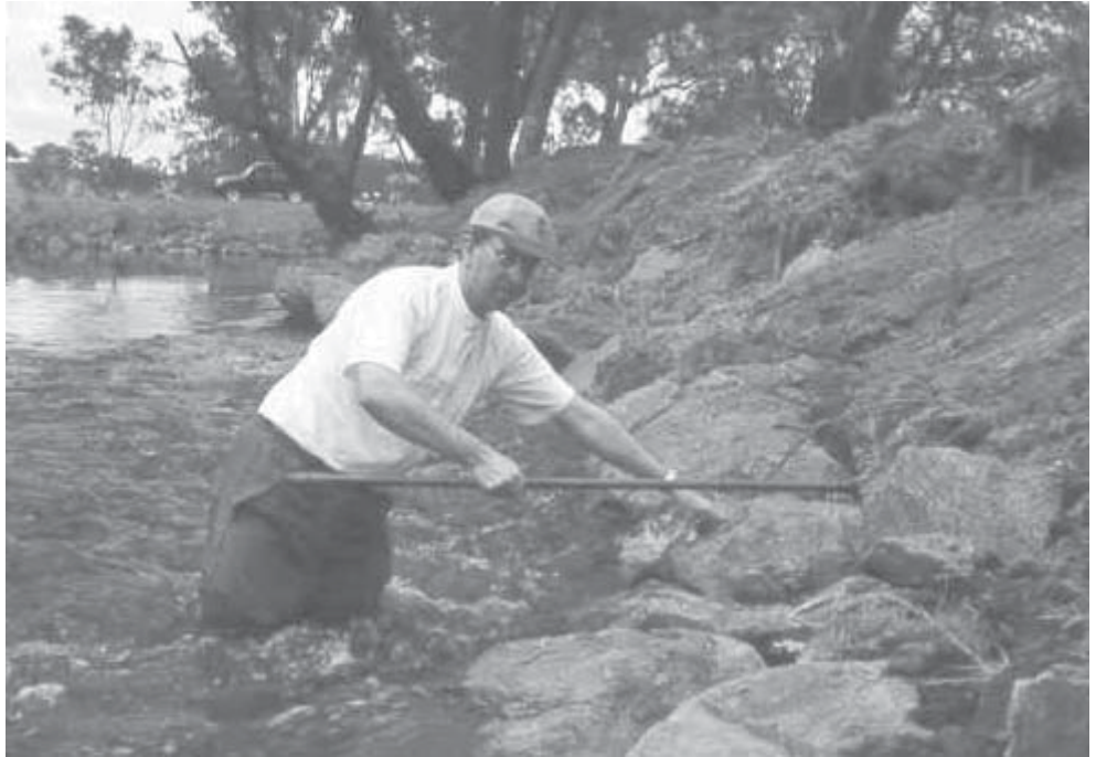
Paul Brown, DPI Victoria, showing the extent of undercut beneath a newly installed lunker [Photo courtesy of Paul Brown]
