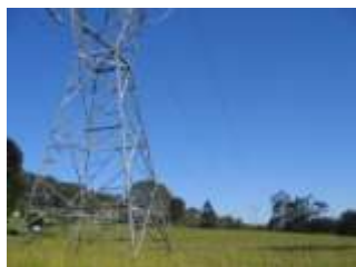
Powerlink transmission lines cross sensitive riparian areas along their route.
