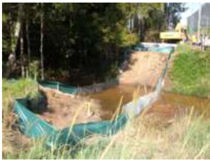
Making the best of an awkward situation – protecting endangered frogs while installing sewerage pipes.
