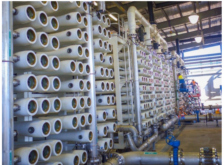
Maintenance work conducted in the Luggage Point Advanced Water Treatment Plant's reverse osmosis room. Image courtesy of Seqwater
