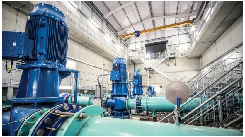
New pumping station – Courtesy of Essex and Suffolk Water
