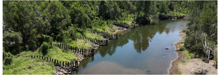
Above: Upper Mary Catchment pile field helping stabilise eroding banks, improve channel stability and support riparian vegetation recovery.
