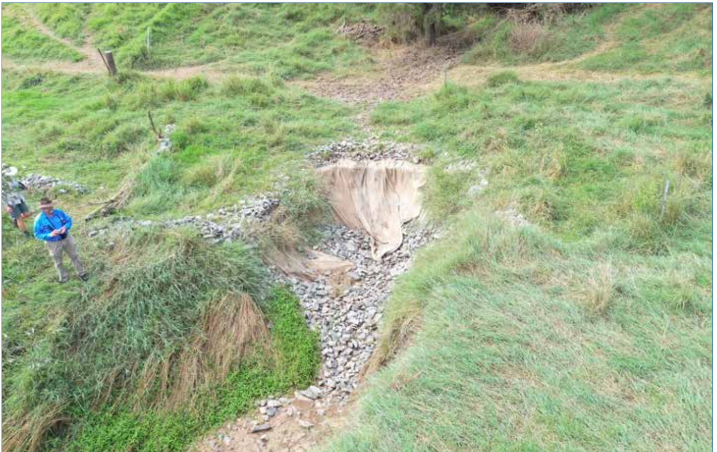
Photo 128 February 2022, after major flooding in the area.
