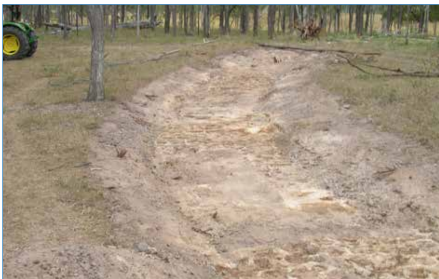
Photo 57 Main diversion bank level sill outlet.
