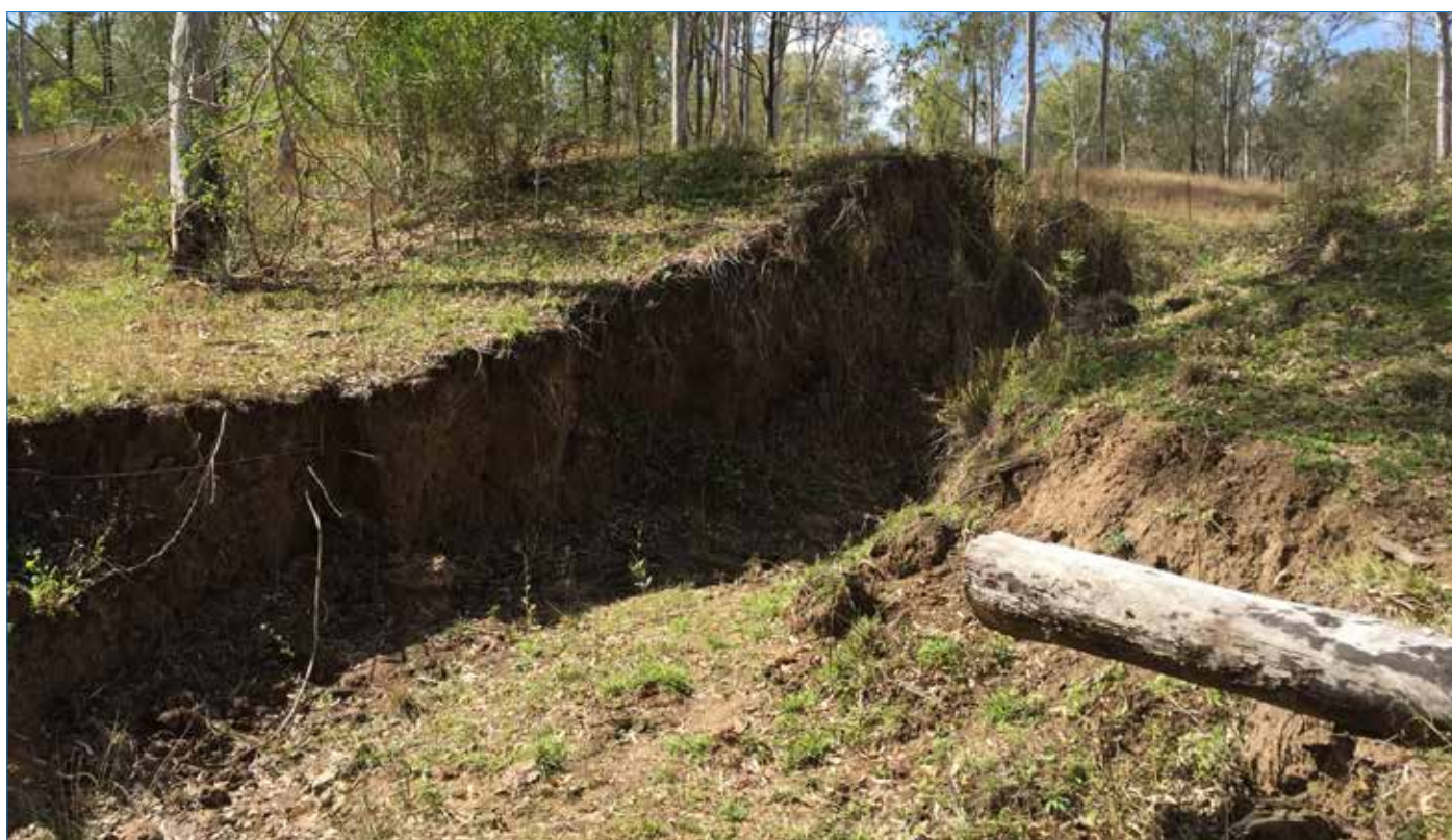
Photo 88 Break in dam wall prior to work.
