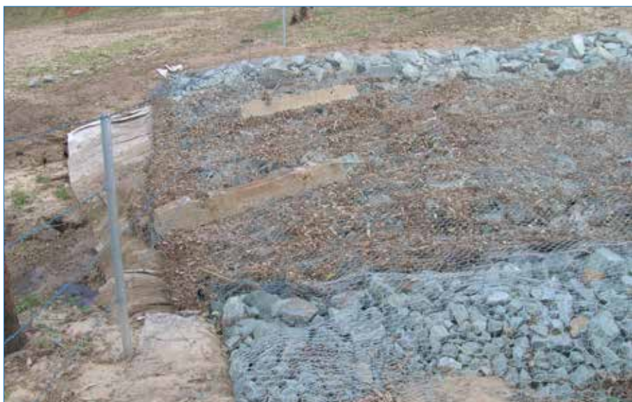
Photo 99 Downstream end of the mattress after the first rain event.
