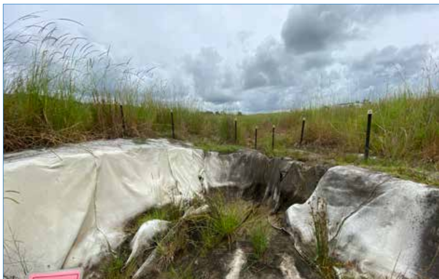
Photo 136 February 2021 monitoring, following two wet seasons.
