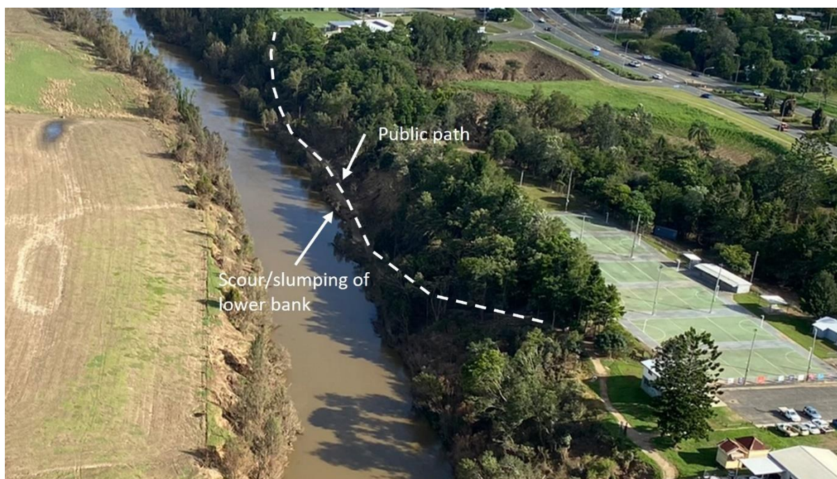
Figure 33. Erosion of lower bank adjacent to public walking track in the lower portion of Sub-reach 2
