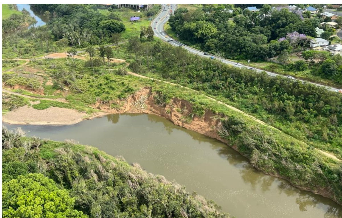
Figure 38. Example of section of bank with a very high erosion potential in Sub-reach 2
