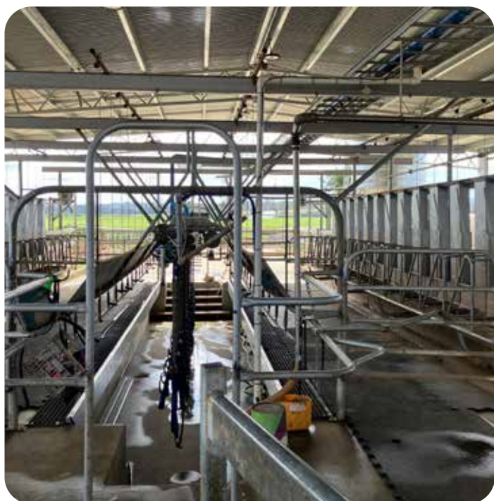
Newly installed herringbone dairy for the Kahler's 145 or so milking cows chosen to minimise waste during milking
